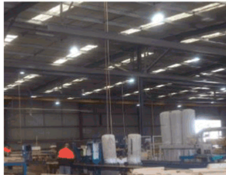
Figure SC21 New energy efficient lighting at Peuker and Alexander, Campbellfield
