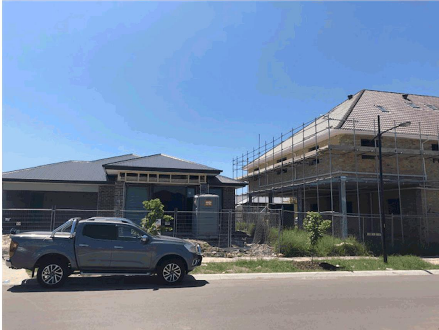
Figure 3 – Facing north towards the neighbouring dwelling at 4 Adventure Crescent and the medical centre currently under construction at 50 Arena Avenue (dated 30 October 2019)
