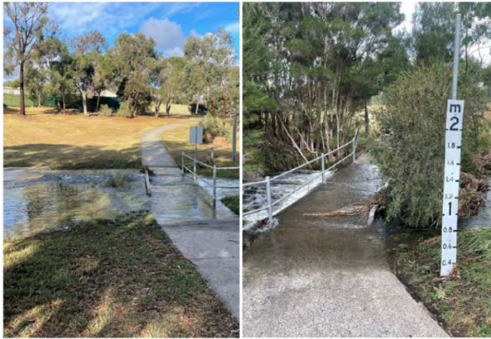
Photo 5. Flooding of low bridges is a regular occurrence after rainfall
